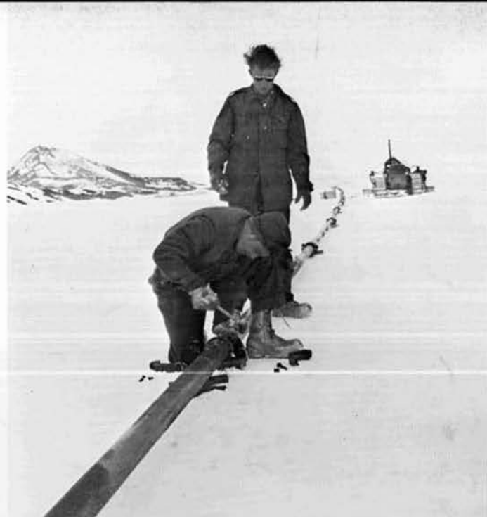
The Pipe line is laid on the bay ice from Hut Point to the prospective berthing site. The oil cargo will then be pumped from the ships to the storage tanks on Hut Point.
