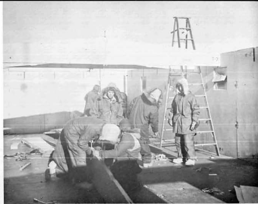
Also brought in on the C-130's were volunteer workers off the CG icebreaker EASTWIND and the USS ARNEB, AKA-56 (above) These men helped erect T-5 type buildings at the Pole Station (left).
